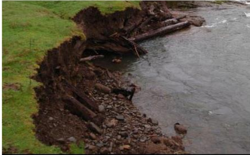
Fig. 3.5. Stream bank erosion. (Source: www.sswc.org )
