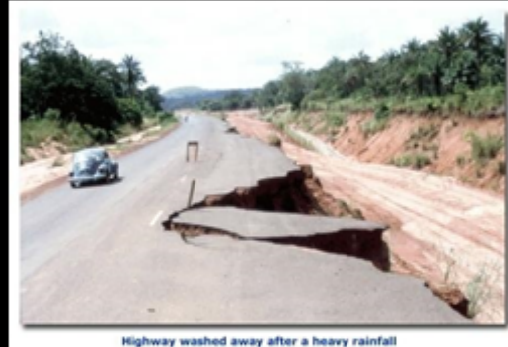
Highway washed away after a heavy rainfall
